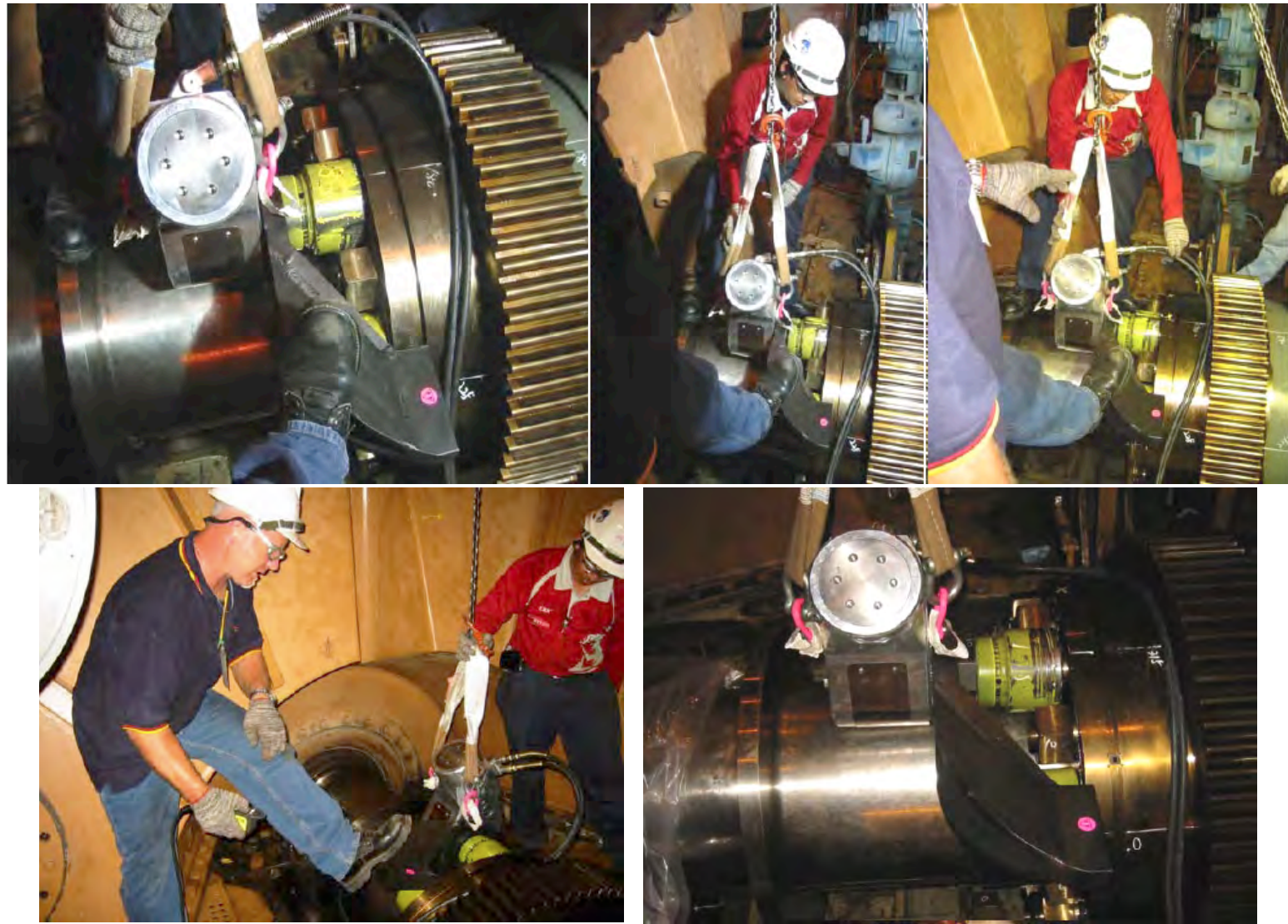
ABOVE PICS: GE 460MW coal fired Steam Turbine, AVANTI-50 used to break out the 4-1/4" nuts on the A & B stage Turbine Coupling bolts.
